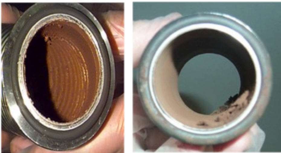
Figure 2- Examples of fully reacted amorphous silicon dust visible in the portions of the exhaust plumbing during a cleaning process.
