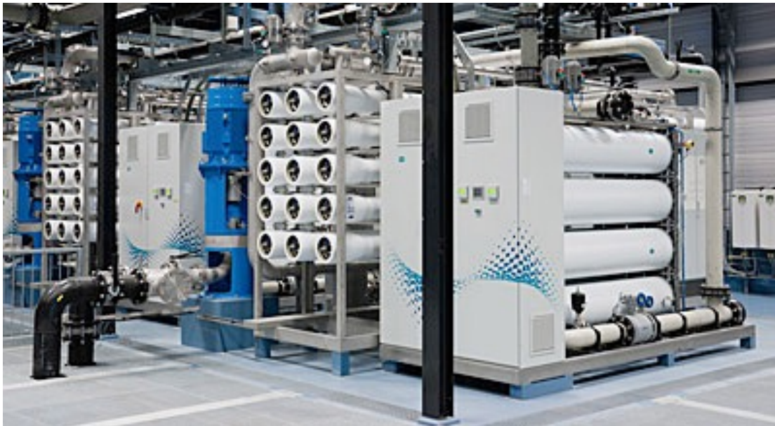
Figure 2- In-house Ultra-Pure Water (UPW) generation system.
