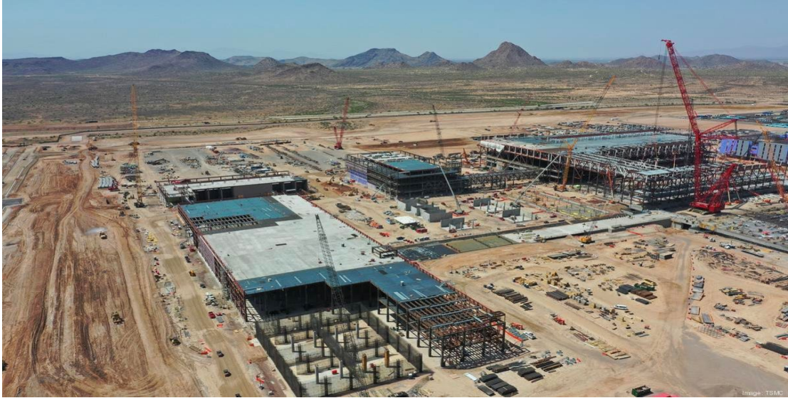
Figure 6- Photo of the TSMC fab in north Phoenix during its construction phase
