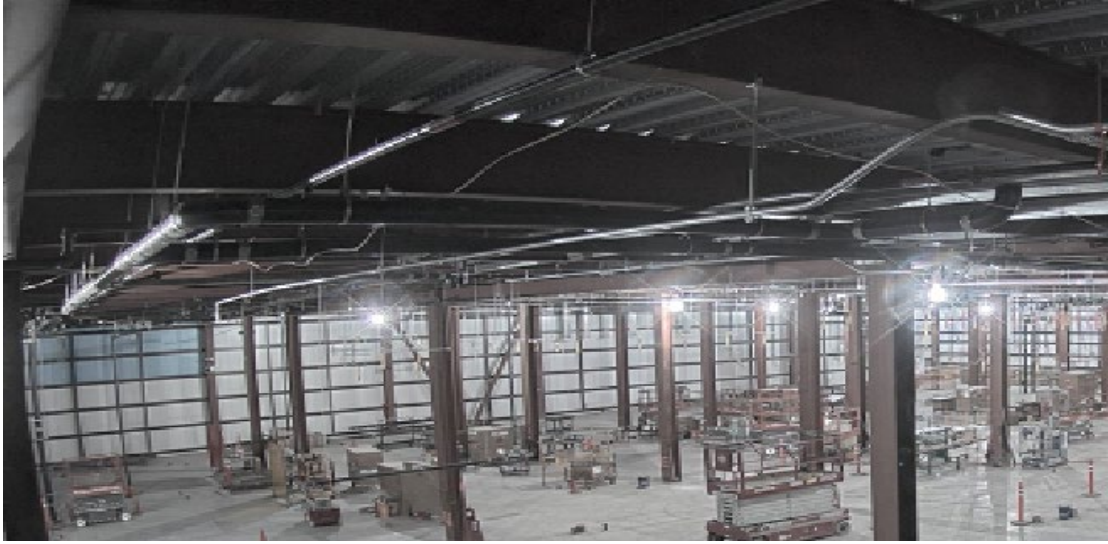
Figure 4- Photograph of the inside of a cleanroom area during the construction phase
